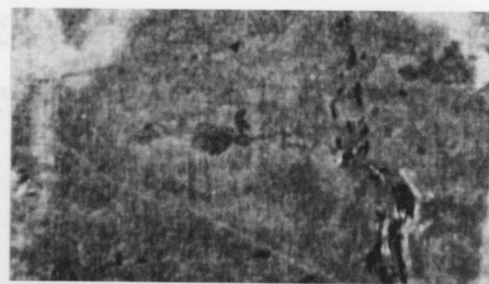
(a) Isolated crack
